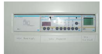
Above: Hager, Tebis switchgear in the installation
